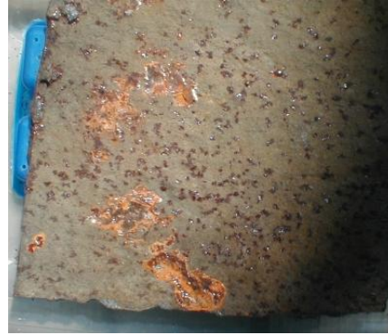
Figure 6 Marine Steel UHP WJ Cleaned Exposed to Humidity 6 years later
